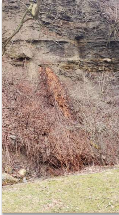
PHOTO 1: Acid mine drainage along WV-88
